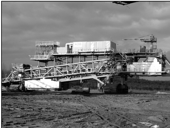
Fig. 4. Container based on air-conditioned e-houses for MV-, LV-switchgears and converters as a basis for minimised downtime during the refurbishment and reduced maintenance efforts during operation of mining devices
