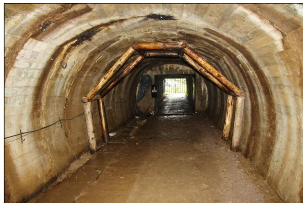
Fig. 2. Podgórze uranium mine in Kowary—conservation works inside the shaft through implementation of polygonal wooden support to the space reinforced and secured with a concrete arched support; photo by T. Wieja.
