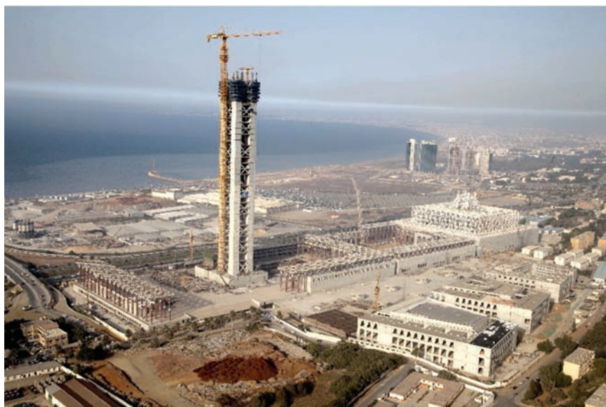
Ill. 9. The new Grand Mosque of Algeria (Djamaâ El Djazaïr) under construction. Source: https://www.kuk.de/ru/proekty/vysotnoe-stroitelstvo/detail/Projekte/show/djamaa-el-djazair-grosse-moschee-von-algier.html (accessed:28.03.2020)
