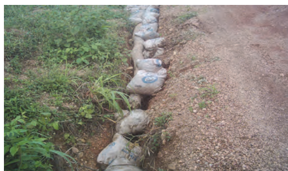
Photo 5. Packs of sand bags as erosion control measures in the study area (phot. O.A. Lawal-Adebowale)
