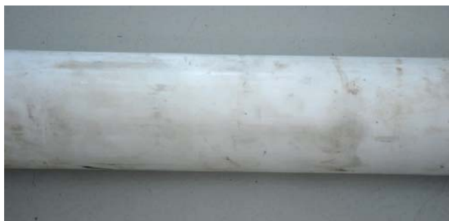
Fig.12. Condition of CTP pipe protection layer after tests – no outer layer damages
