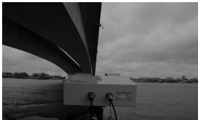
Fig. 9. Dynamic load tests of long reinforced concrete spans exemplified by a bridge near Grudziądz
