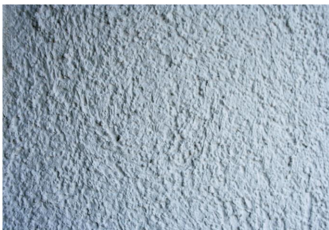
Fig. 4. Skim-coating reinforced with fibre glass mesh, painted with façade paint. Source: Fot. K. Słuchocka
