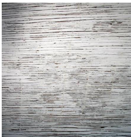
Fig. 3. A wicker mat and mortar that form a wall cladding Source: Fot. K. Słuchocka
