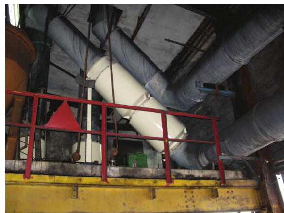
Fig. 3. Example of implementation of variant II of acoustic silencers to the industry (PIERCHALA et al. , 2010).
