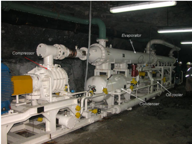
Fig. 2. GMC-1000 Cooling Unit
