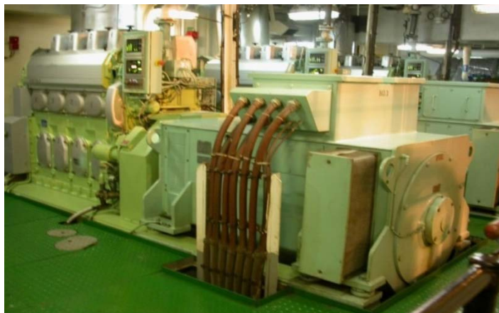
Fig. 1. Electric power generating sets with engines type 4L20D2 made by Wärtsilä
