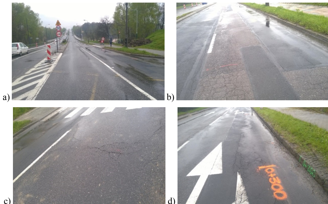
Figure 2. Fragment of Matuszczyka Street in Wodzisław Śląski a) general view, b) mesh patches and cracks in the pavement, c) transverse crack, d) longitudinal crack (own elaboration).
