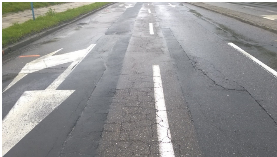
Figure 3. Patches and cracks on the section (0 + 300 - 0 + 400) of the tested road (own elaboration).
