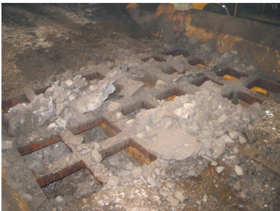
Fig. 5. Grate after URB/ZS-3 has automatically cleaned it
