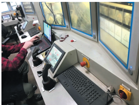
Fig. 3. Remote control console in SK-2 control room on shaft bottom of SW-1 shaft
