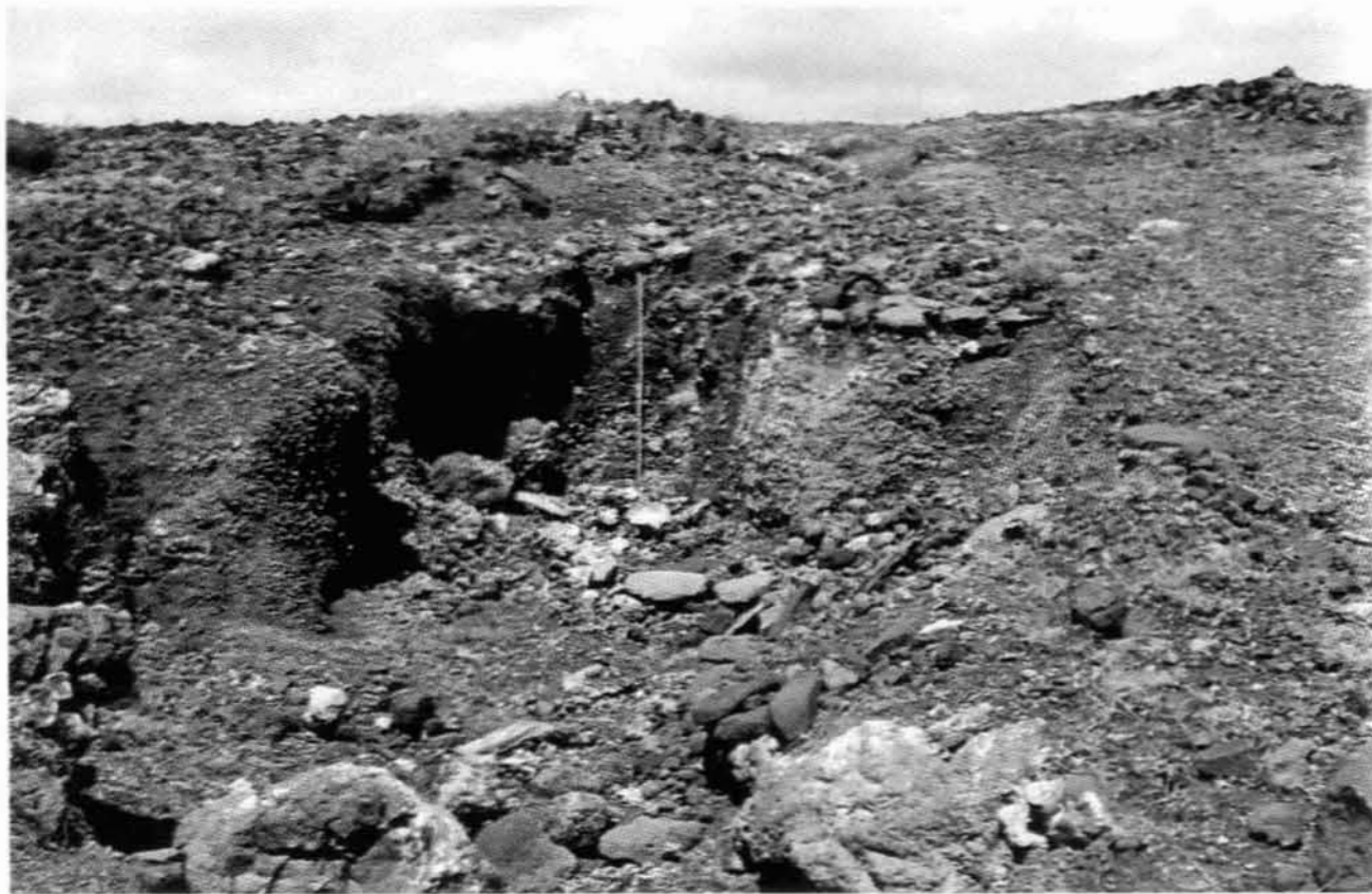
Fig. 7. Eversion hole in the cutting of the unpaved road
