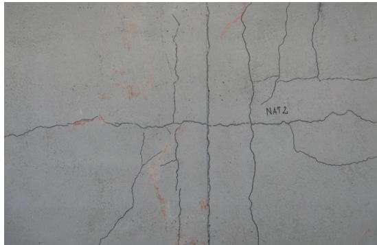
Fig. 7. Experimental cracks for the control slab N.
