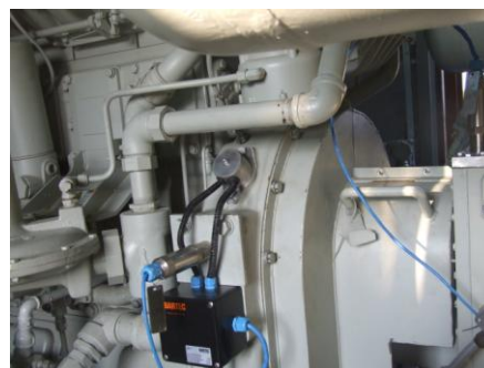
Fig.7. Inductive sensors mounting location and junction box
