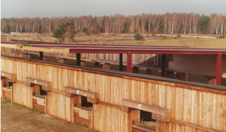
Picture 1. Bulletproof roof over screens P1 and P2 of the experimental shooting range
