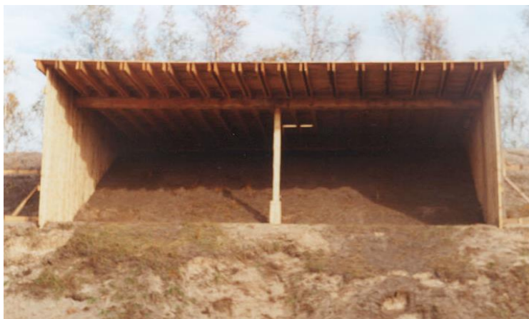
Picture 3. Main backstop of the experimental shooting range, intended to capture ricochets occurring at the bottom backstop, before the main backstop, and on the head slope of the main backstop
