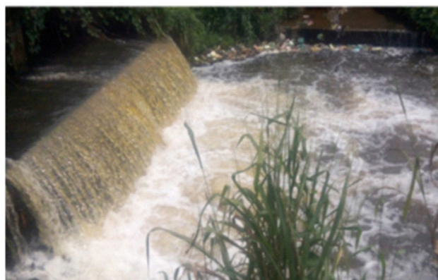
(b) Culvert ending creates a fall in the channel
