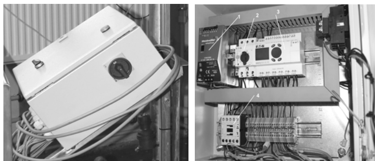
Fig. 3. A general view and the interior of the control cabinet: 1 – 24 V power supply, 2 – motor protection – circuit breaker PKZ-type, 3 – PLC 819-AC-RC 115/240 V / AC, 4 – motor contact
