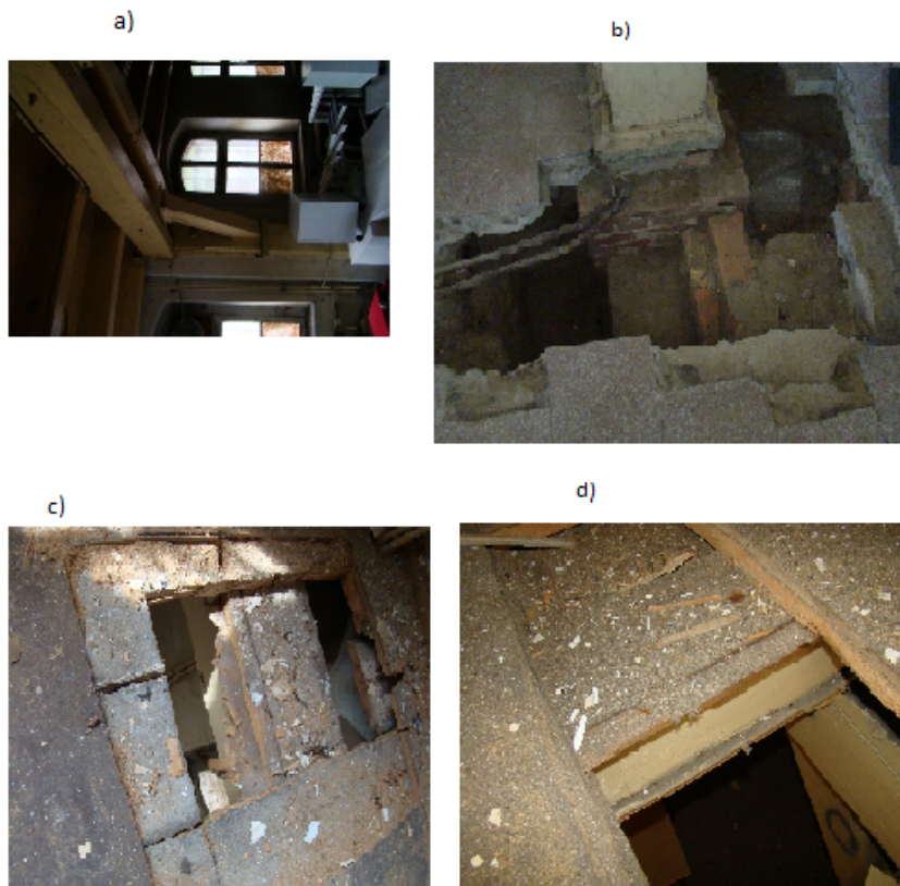
Figure 7. Building planned for modernization ceiling above the ground floor: a) fragment of the wooden frame, b) foundation of the column, c), d) structure of the stop
