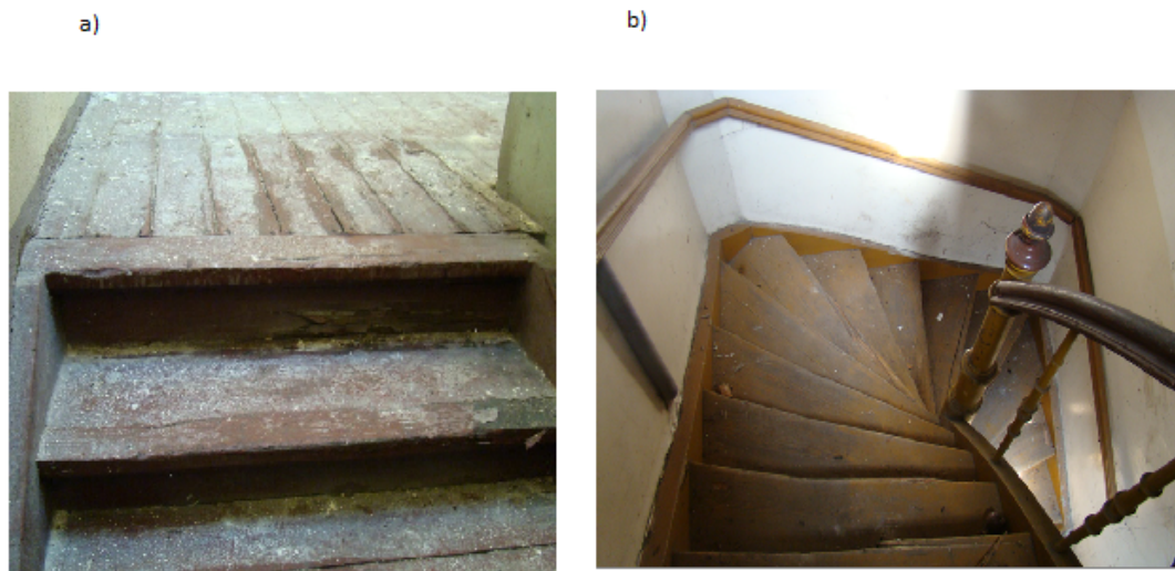
Figure 11. Building planned for modernization - damage to the runs of staircases: a) main and b) side
