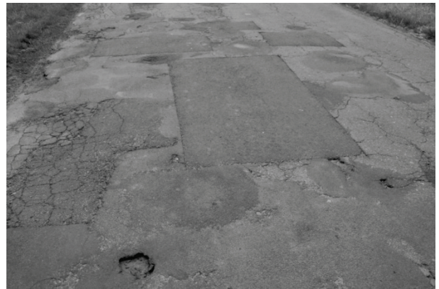
Fig. 4. View of repairs, made of different kinds of bitumen [Own photograph].
