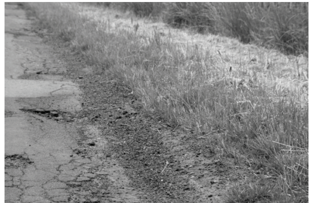
Fig. 5. View of damaged roadside [own photograph].
