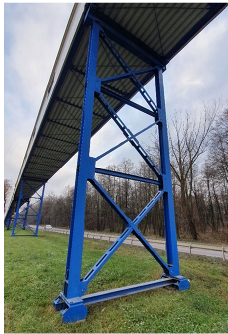
Fig. 6. Swingarm support structure
