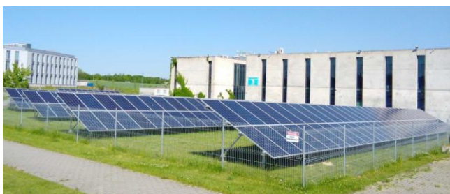
Fig. 2. Photovoltaic plant in front of the building of the Lublin Science and Technology Park [33]
