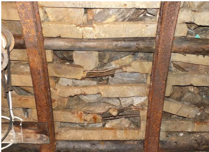
Fig. 1. Damaged reinforced concrete lining
