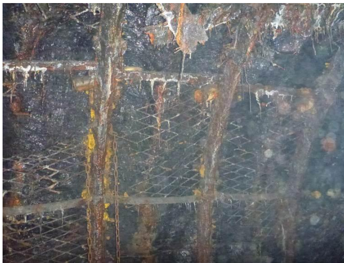
Fig. 2. Corroded MM mesh lining
