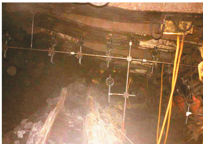
Fig. 2. The discussed section with visible sensors of the multi-point system for methane velocity and concentration measurements
