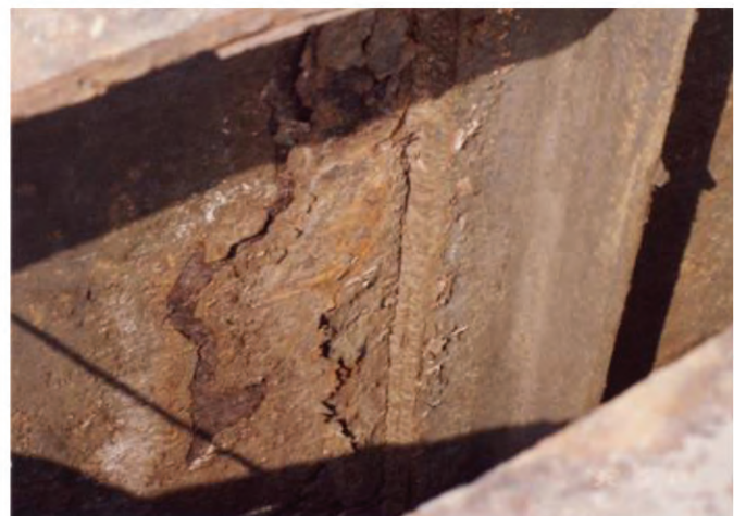
Photo 5. View of the web of a plate girder of a main road bridge – visible fatigue cracking within the welded joint as a result of additional corrosion weakening of the section in the contact zone of the elements
