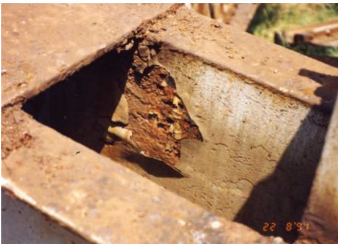
Photo 4. View of the bottom flange of a truss girder of a railroad bridge – visible cracking of the roll-formed section caused by advanced pitting corrosion
