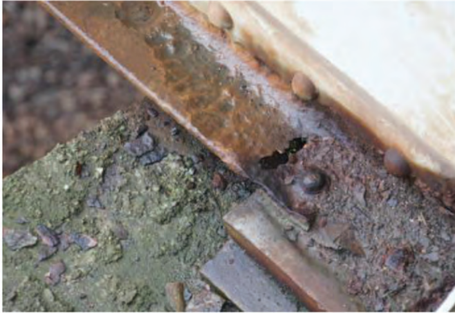
Photo 2. View of the support zone on the bearing of the bottom flange of the main girder of the road bridge – total perforation of the bottom flange due to pitting corrosion can be seen
