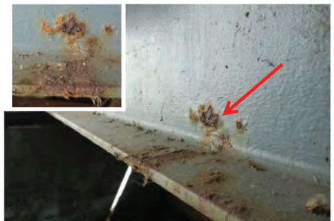
Photo 1. Example of a steel girder of an in-service steel bridge with locally damaged paint coating resulting in pitting corrosion of the structural steel
