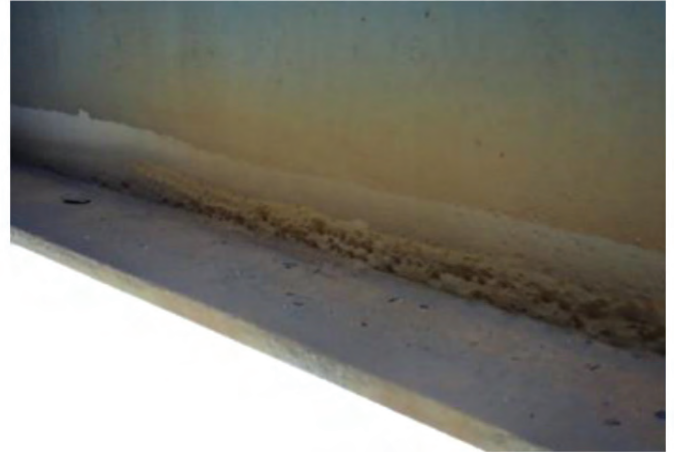
Photo 3. View of the connection zone between the web and the bottom flange of the sheet metal girder of a main railroad bridge – a clearly visible example of the occurrence of pitting corrosion of structural elements, due to the presence of rainwater moisture
