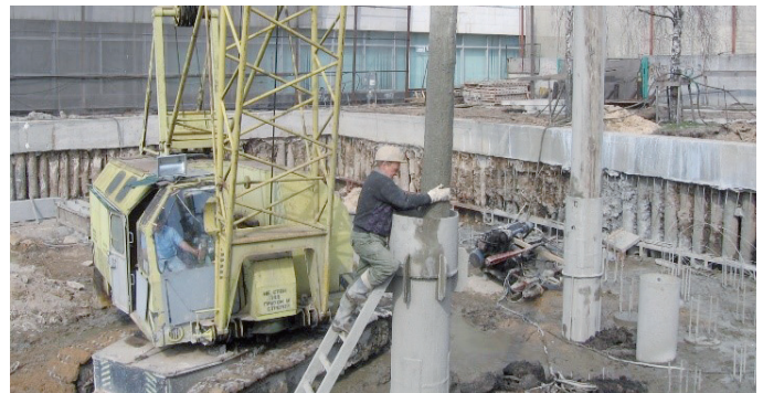
Figure 4. Structure of bored piles in saturated sands: on the left – installation the bailer for excavating from the casing of biogenic soils over the compacted ground plug to the right – its displacement by a second pipe with closed end
