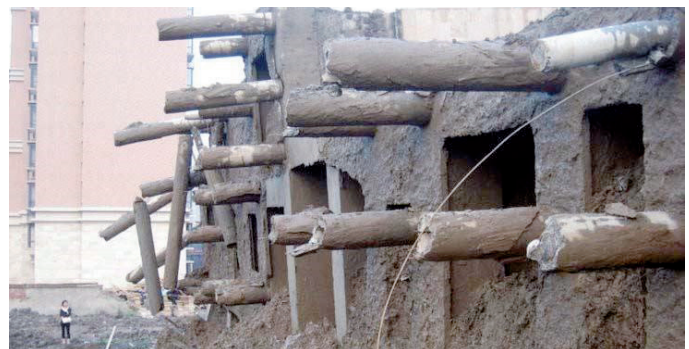
Figure 3. Collapsed in Shanghai, a 13-storey residential building [24] in the failure of prefabricated hollow reinforced concrete piles, weakly reinforced by tensile rods of small diameters
