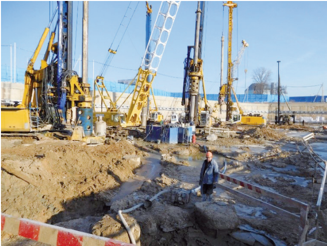
Figure 5. Drilling wells by drilling rigs of the firms «Bauer» and «Cassagrande» under the protection of casing pipes with scooping out of the ground by bailers and refilling of water into the casing
