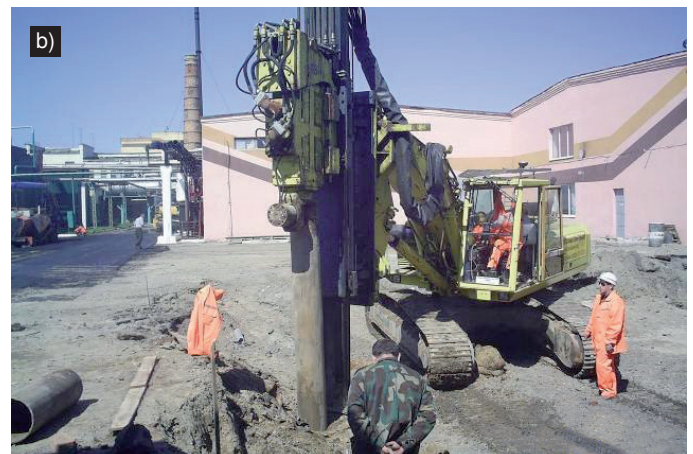
Figure 9. Making holes for bored piles: a – driving conical punch by using hanging vibratory, b – driving cased shaft by vibrating, on the hard track machine ABI
