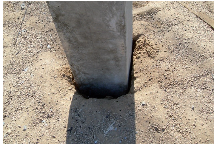
Figure 1. The gap between sandy soil with rupturing cracks in the corners when the pile body is tilted from misaligned hammer impacts during pile driving
