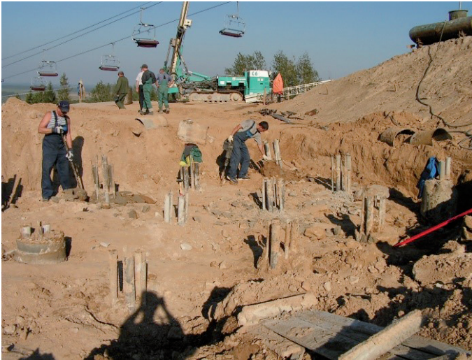
Figure 17. Piles for end support cableway lift snowboard in Silich by inject technology (in the background can be seen the machine company «Kasagrande» to perform pile)
