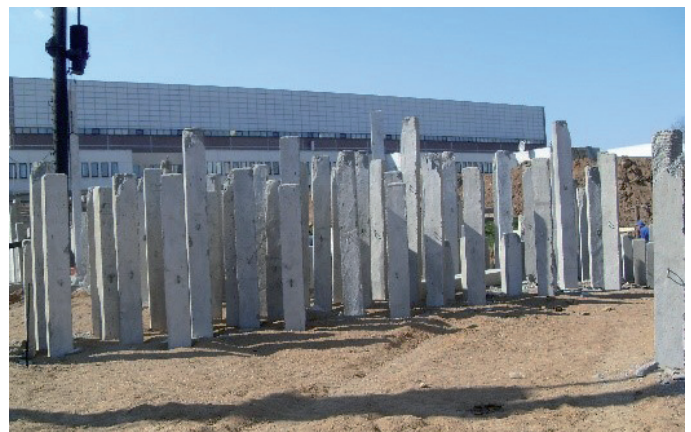
Figure 2. Not be driven to design marks of piles
