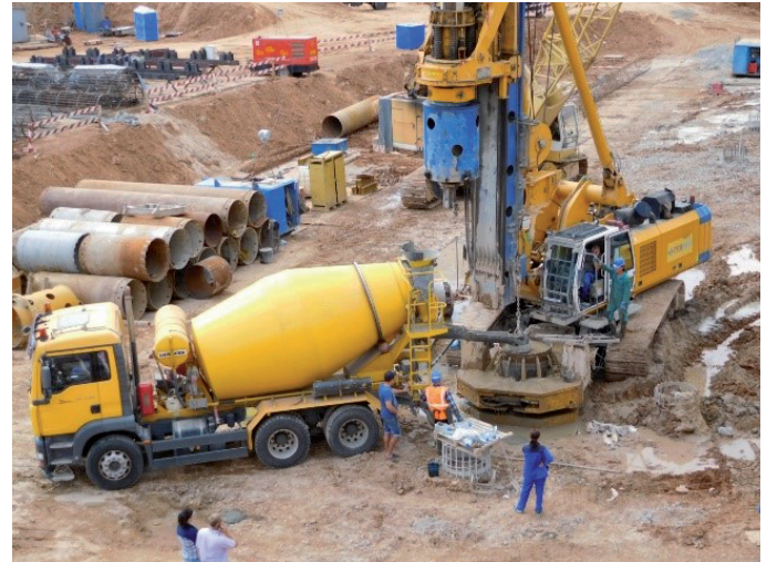
Figure 6. Concreting of piles in a casing filled with water by the method of VPT when pouring concrete from a mixer through the socket of a concrete pipe
