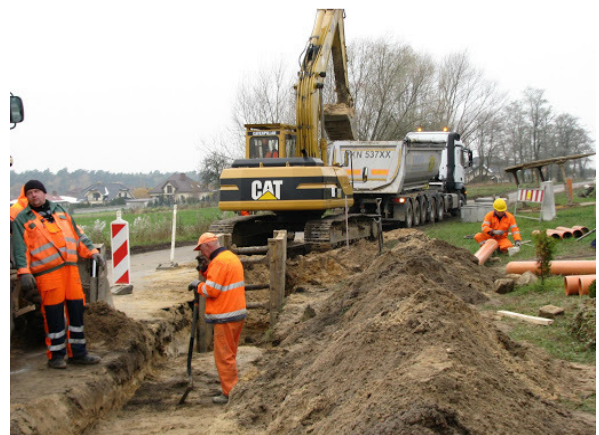
Fig. 1 Example of making sewage system installation using traditional methods with a big number of groundworks Source: [4].
