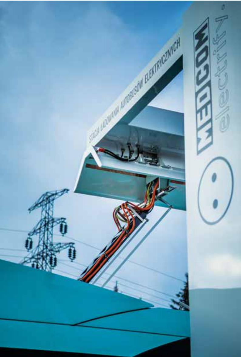
The electric buses charging station made by MEDCOM in PKM Jaworzno
