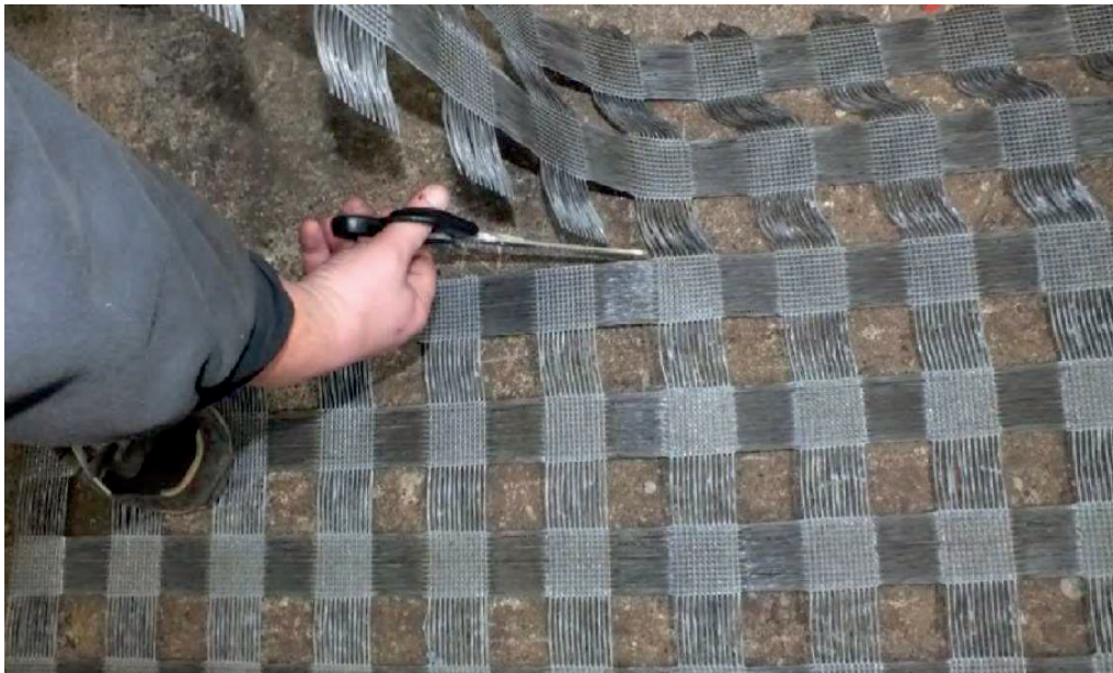
Pic. 3. Cutting the netting on the mine working to the correct size Fot. 3. Przycinanie siatki opinkowej do żądanego wymiaru Source: Materials owned by PPUW Ankara, by courtesy of the company.
