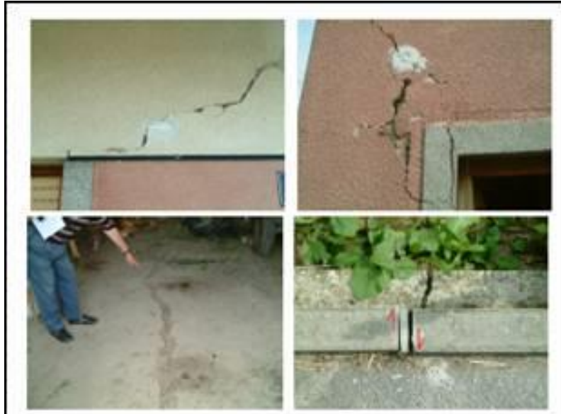
Figure 8. Examples of damages on houses in the epicentral area near Zagreb
