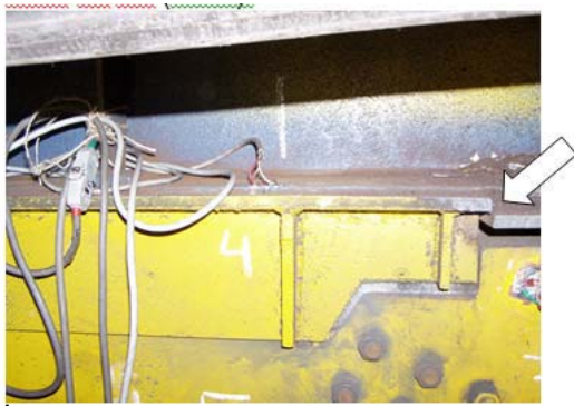
Fig. 8. Photo-documentation of a fatigue crack, side view
