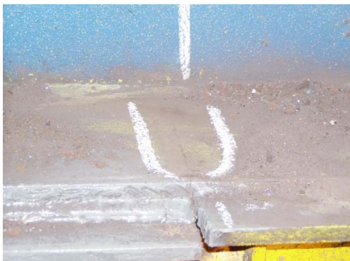
Fig. 9. The same fatigue crack, view from above
