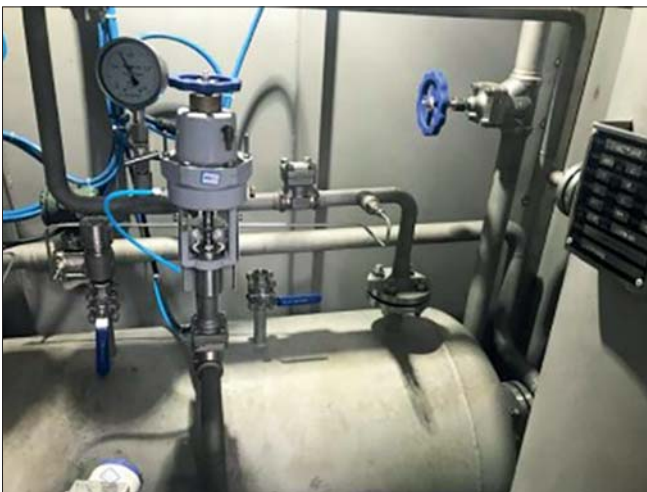
Fig. 2(a). Spiral-wound heat exchanger
