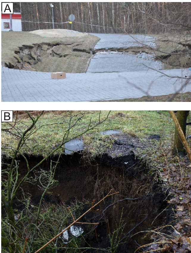
Fig. 2. Sinkholes at Rybno
