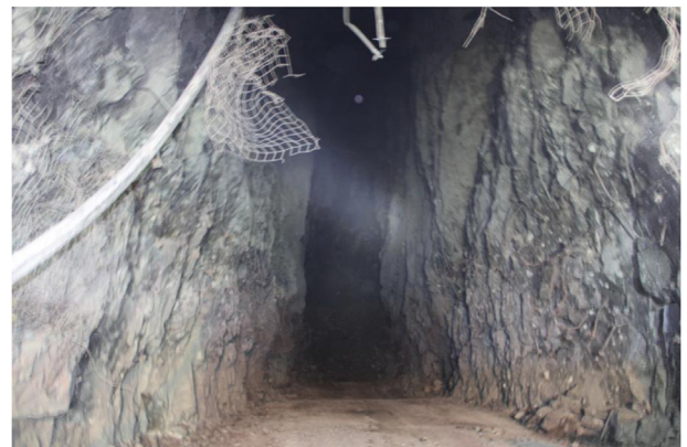
Fig. 5. View of a typical open stope at the analyzed underground diamond mine.
