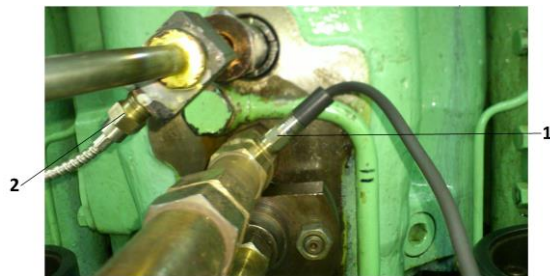
Fig. 1. The research with the engine SULZER 3AL25 / 30 - view on one of the cylinder cover with converters installed with an electronic indicator co-operating: 1 - 6353A24 Kistler sensor for the measurement of cylinder pressure; 2 - sensors for measuring pressure in the injection system's Optrand AutoPSI type-S
