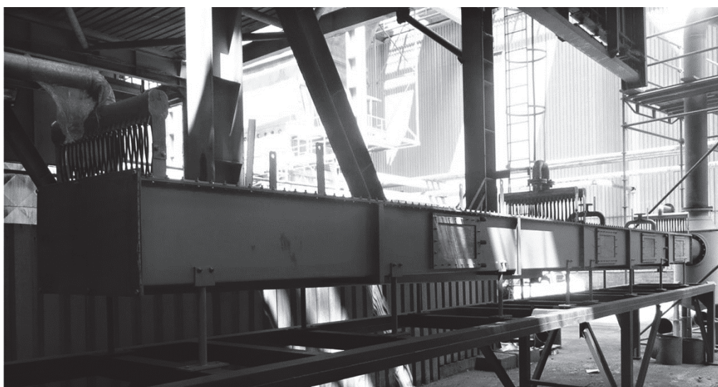
Fig. 4. View of the heat exchanger during the installation at the pilot-scale plant
