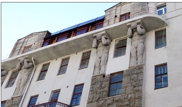
Fig. 2. A fragment of the facade of the former building of the Kharkiv City Commercial (Merchant) Bank and the Astoria Hotel, current state; photo by O. Remizova.
