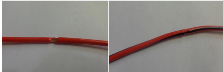
Fig. 5. Cable with damaged insulation.
