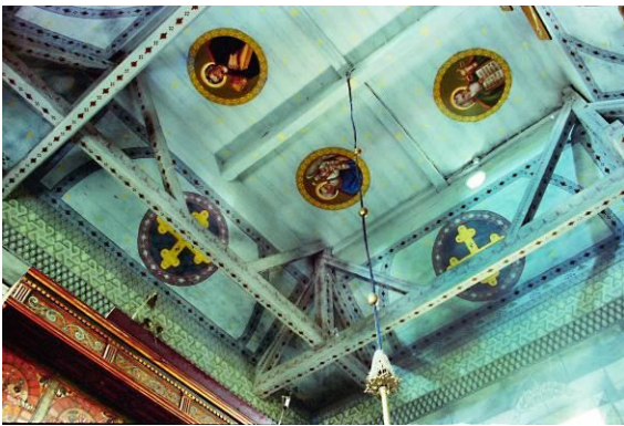
Fig. 15. With larger spans of the nave covers, its structure requires the introduction of additional structural reinforcements. Source: photo author
