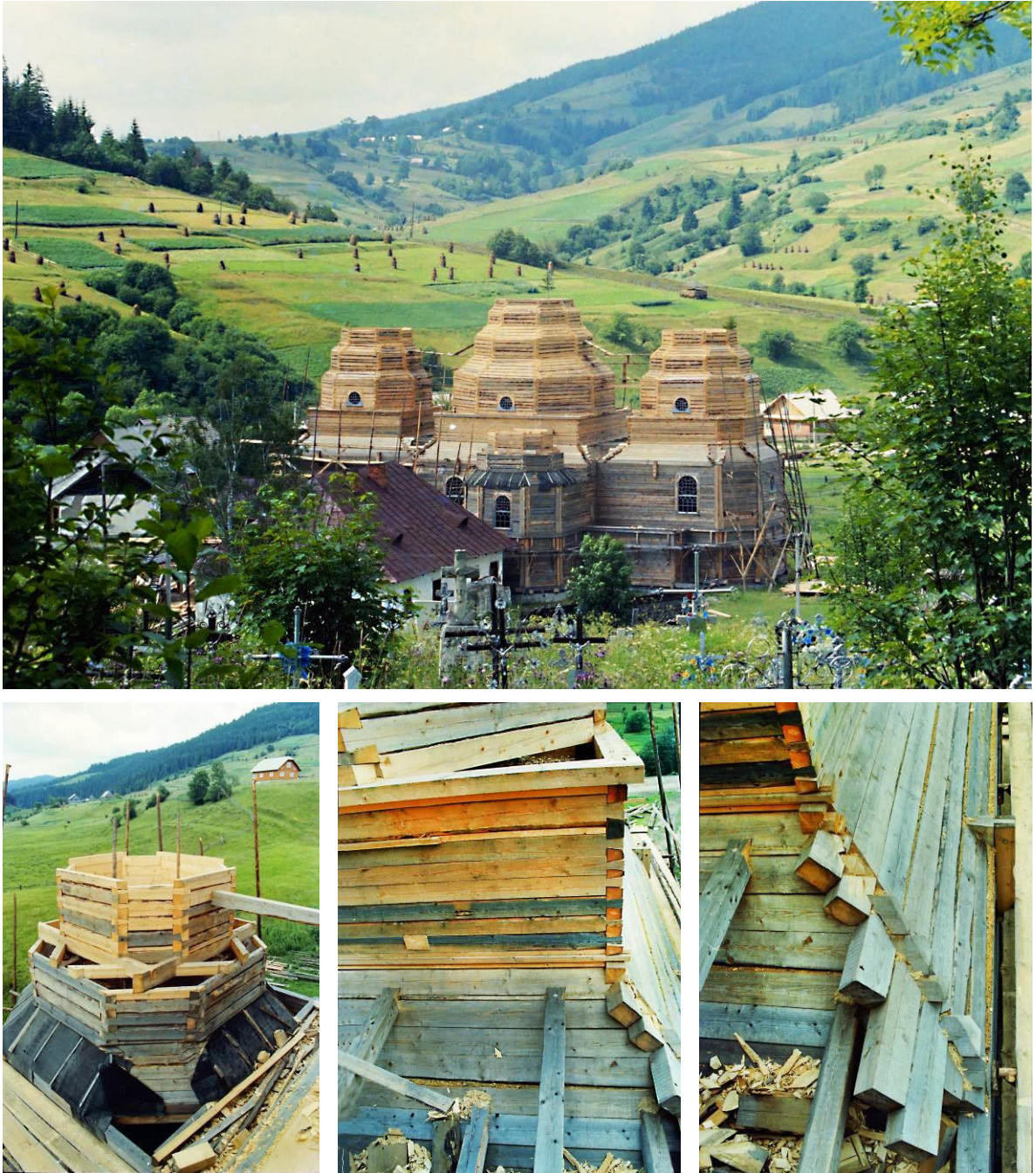
Fig. 17. In the foothill region of the Carpathians, until the end of the 20th century Orthodox churches were built according to traditional structural and formal patterns – e.g. in Wolosianka. Source: photo author 1996
