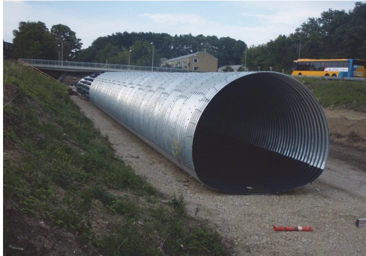
Figure 7. Assembled structure – bottom section painted with bitumen. The ramp on the left
