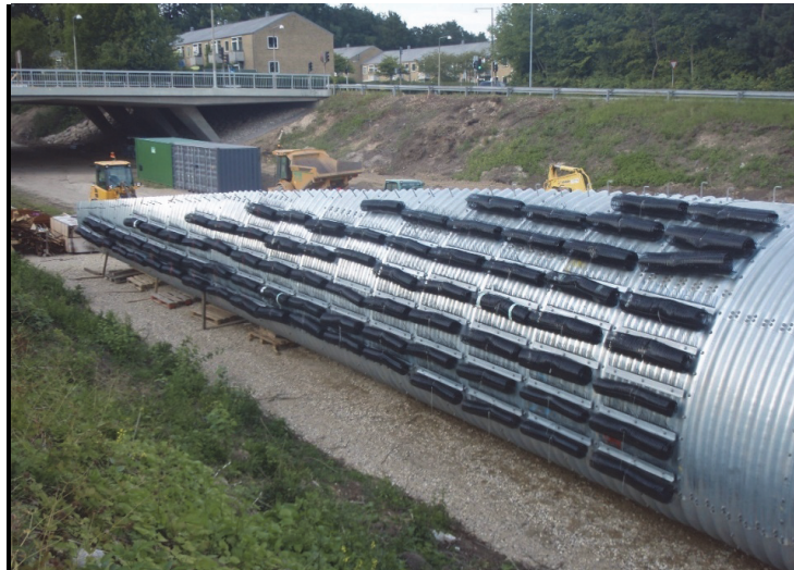
Figure 9. The 21.6 m long bevel end has been provided with geogrid (soil reinforcement)
