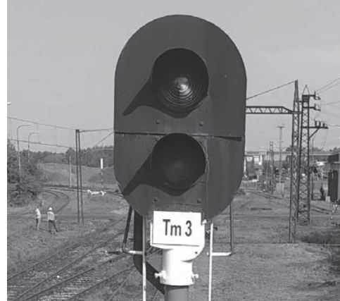
Fig. 6. A shot to test the correctness of the signaling aspects [own study]
