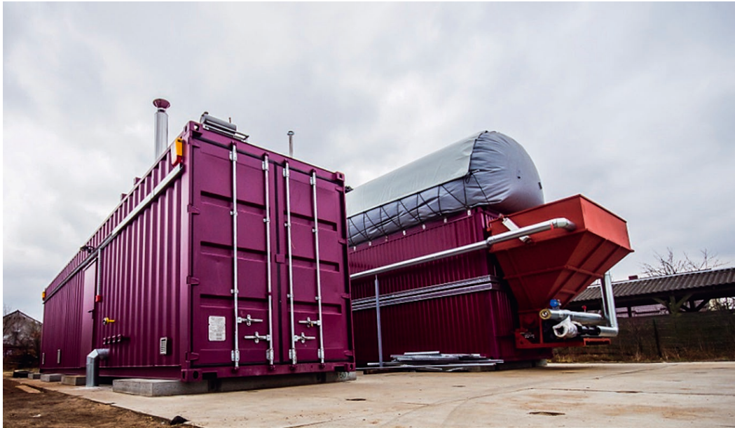
Photo 1. 10 kW container biogas plant (photo by the author)
