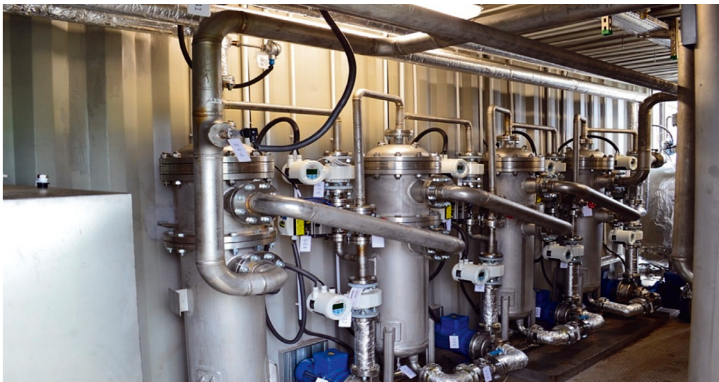
Photo 2. Container biogas plant with 200 m 3 /h SFR reactors (photo by the author)
