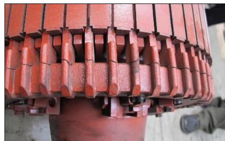
Fig. 3. Damaged rotor winding of traction machine.
