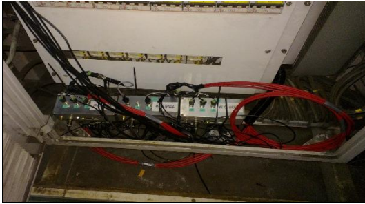
Fig. 7. Telemetry, multi-channel data acquisition system mounted in the switchgear of the rail vehicle.
