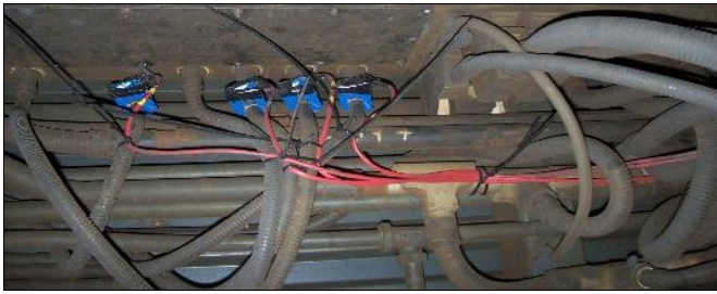
Fig. 6. Current transducers mounted under the rail vehicle.
