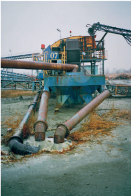
Fot. 5. Burzliwe przelewy z obu odwadniaczy, ucieczka piasków do osadnika. Wariant III Photo 5. Turbulent overflows from both dewaterers, escape of sands to settling tank (option III)
