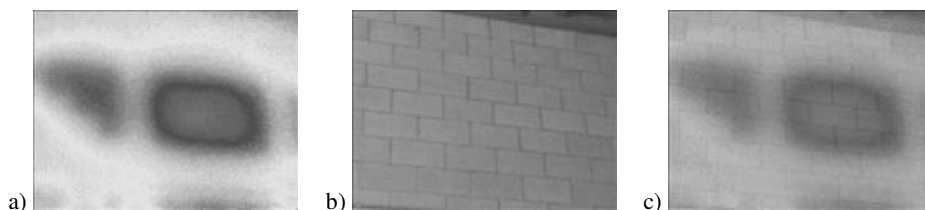
Fig. 11. Example of location of missing filling in a wall of bricks: a) the image captured with IR camera, b) image captured with VIS camera c) fusion of images with the set value of diffusion of 50% (identification of defects) [9]
