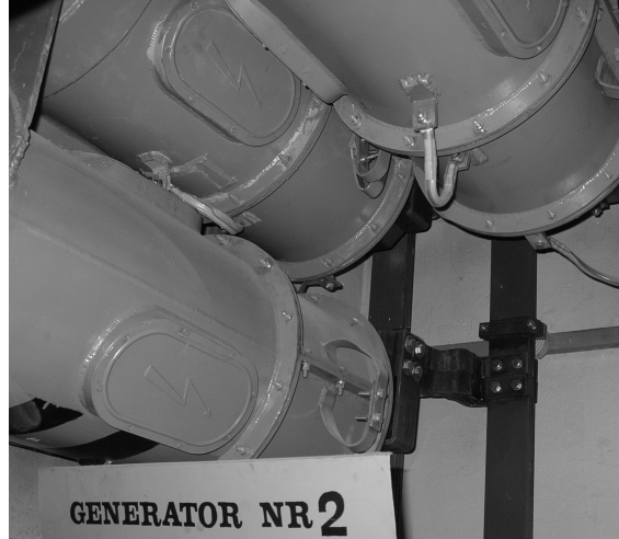
Fig. 4. High current busduct in the power plant. Reproduced by permission of Holduct Ltd [10]
