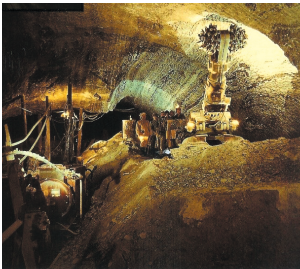
Fig. 1. Use of the AM-50 roadheader in the galleries of the “Ważyn” Chamber (phot. from the collection of the “Bochnia” Salt Mine)
