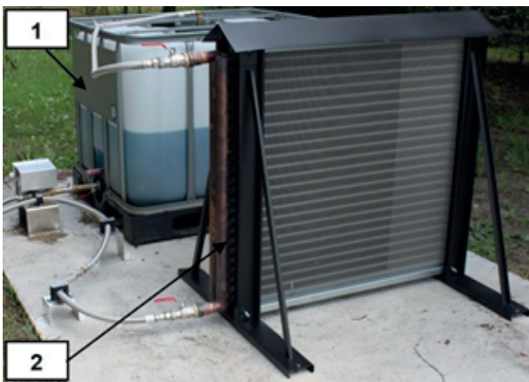
Fig. 6. Elements dispersing thermal energy located outside: 1) external coolant tank, 2) external fanless cooler
