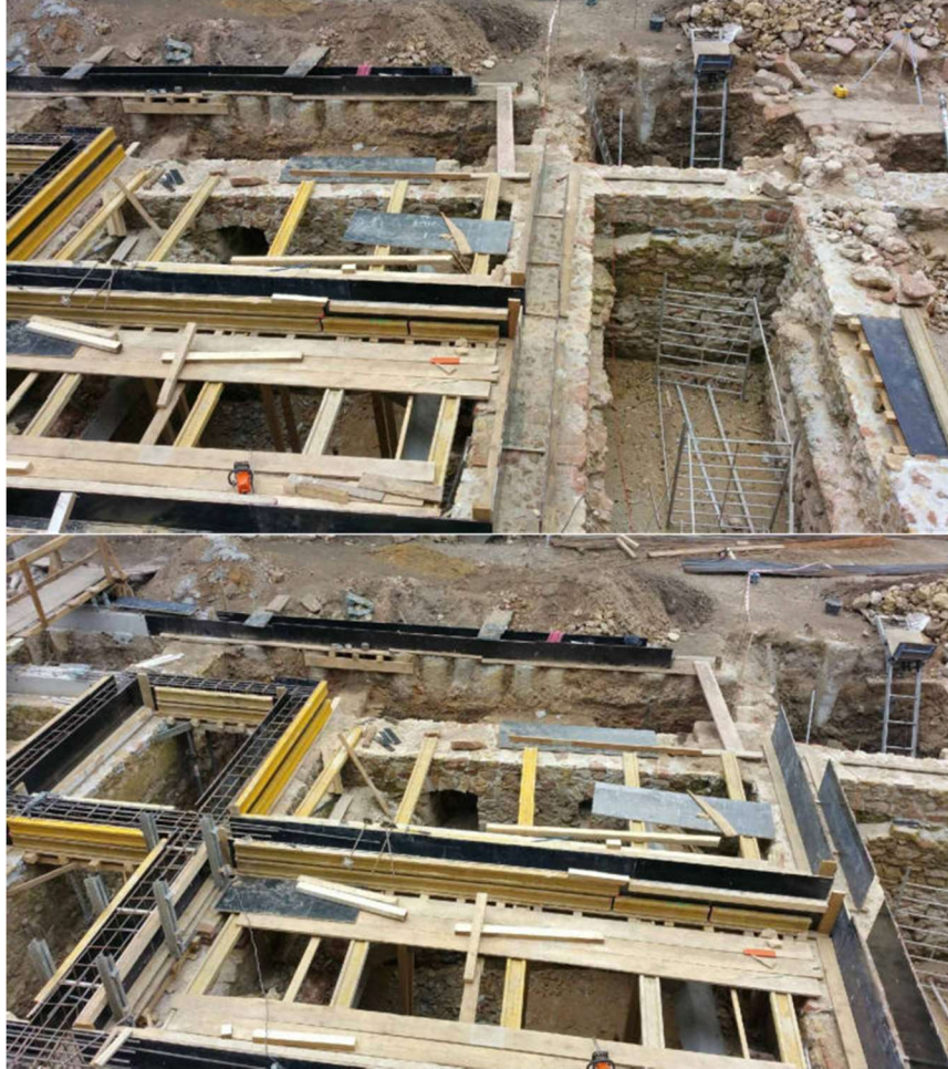
Fig. 13. Construction of the floor slab over the uncovered medieval cellars under the courtyard (Photo by the author)
