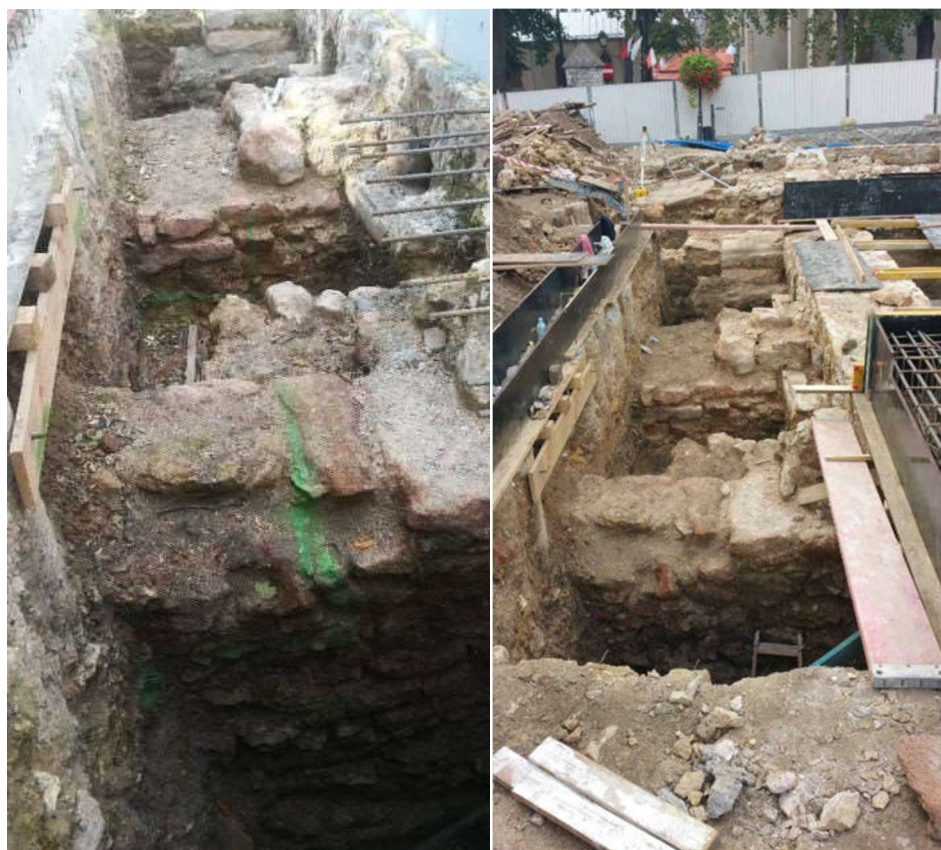
Fig. 12. Construction of load-bearing beams for the courtyard slab (at the same time - the floor slab above the medieval cellars) (Photo by the author)
