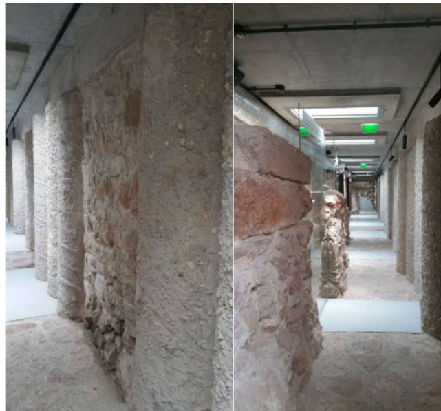
Fig. 19. Cellars under the courtyard, after uncovering and renovation. Palisade retaining wall – detail (on the left). The permanent exhibition rooms, naturally lit by skylights (on the right) (Photo by the author)
