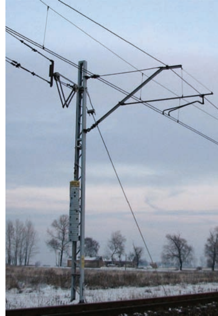
Fig. 1. T-profile catenary equipment and weight tensioning device [photo P. Kwaśniewski]
