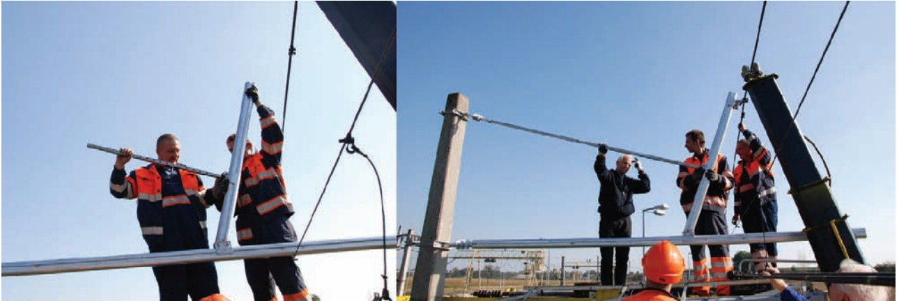
Fig. 24. Assembly of the new OCL cantilever system at IK Test Track Centre near Żmigród [photo P. Kwaśniewski]
