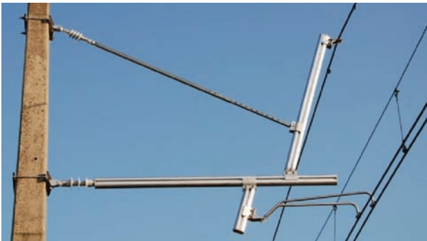
Fig. 25. New OCL cantilever system mounted at IK Test Track Centre near Żmigród [photo P. Kwaśniewski]
